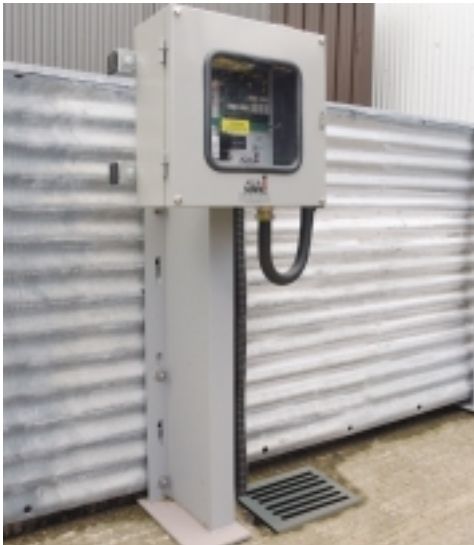
Control Panel (shown installed on bund wall) can be sited at other locations eg. site office.
