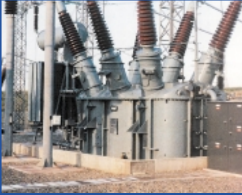
Example of a typical concrete bund containing an oil filled transformer.
